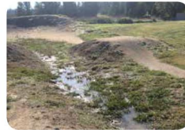
Existing drainage issues
